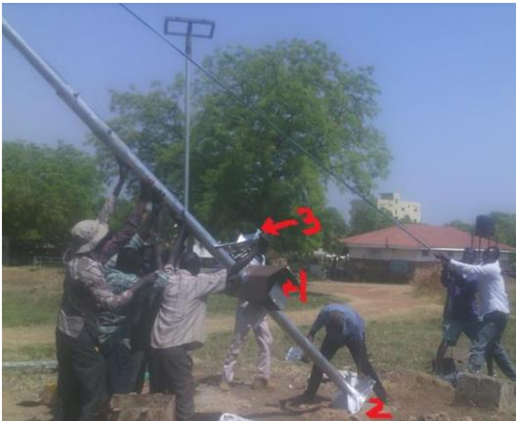
Figure 4.1: Fixing the old 10m pole on the concrete slab with screws and nuts
